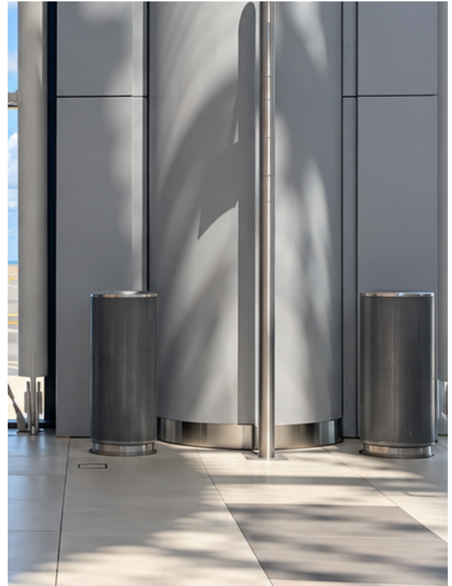
Figure 13. Displacement diffusers integrated beside an airport terminal column.
